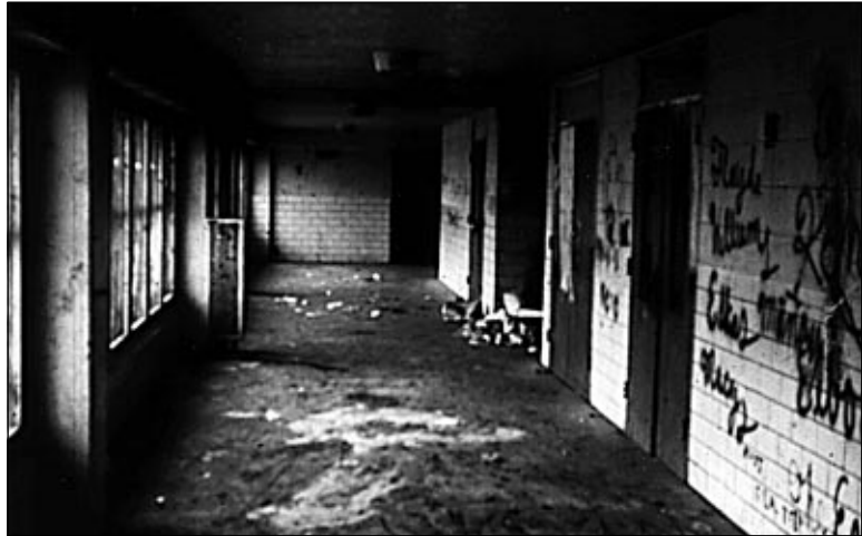
Figure I-3: The 3d floor communal corridor as it actually turned out, showing the vandalism that ensued.
